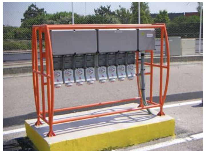
Container Terminal, Le Havre – France
